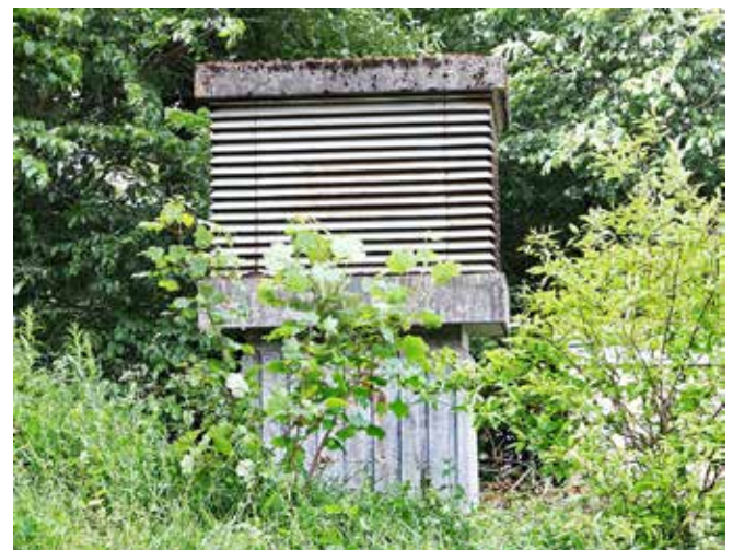
Ventilation stack; slowly being consumed by the overgrowth Newly established as the designated Highland Council Emergency Centre, the bunker would see active use
